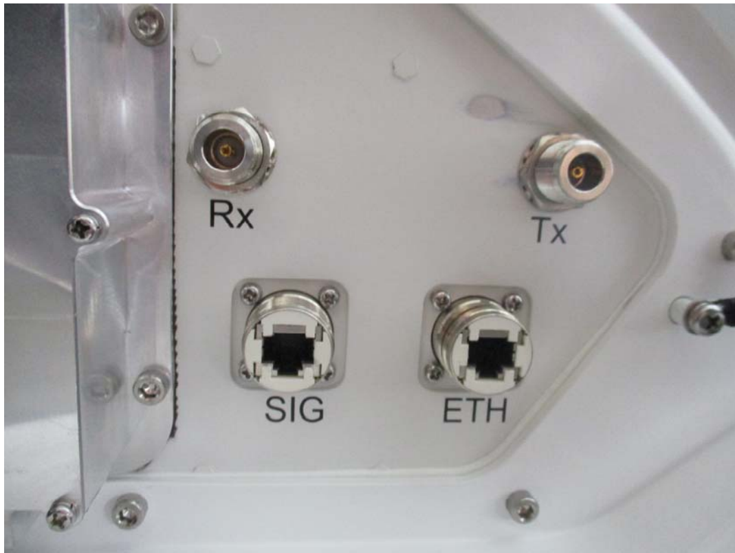
Primary Antenna (located at Bottom of Antenna)
