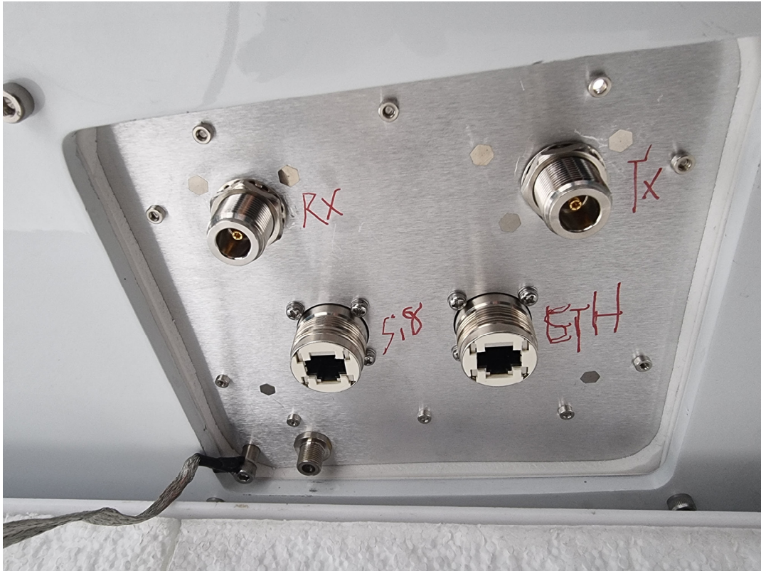
Primary Antenna (located at Bottom of Antenna)
