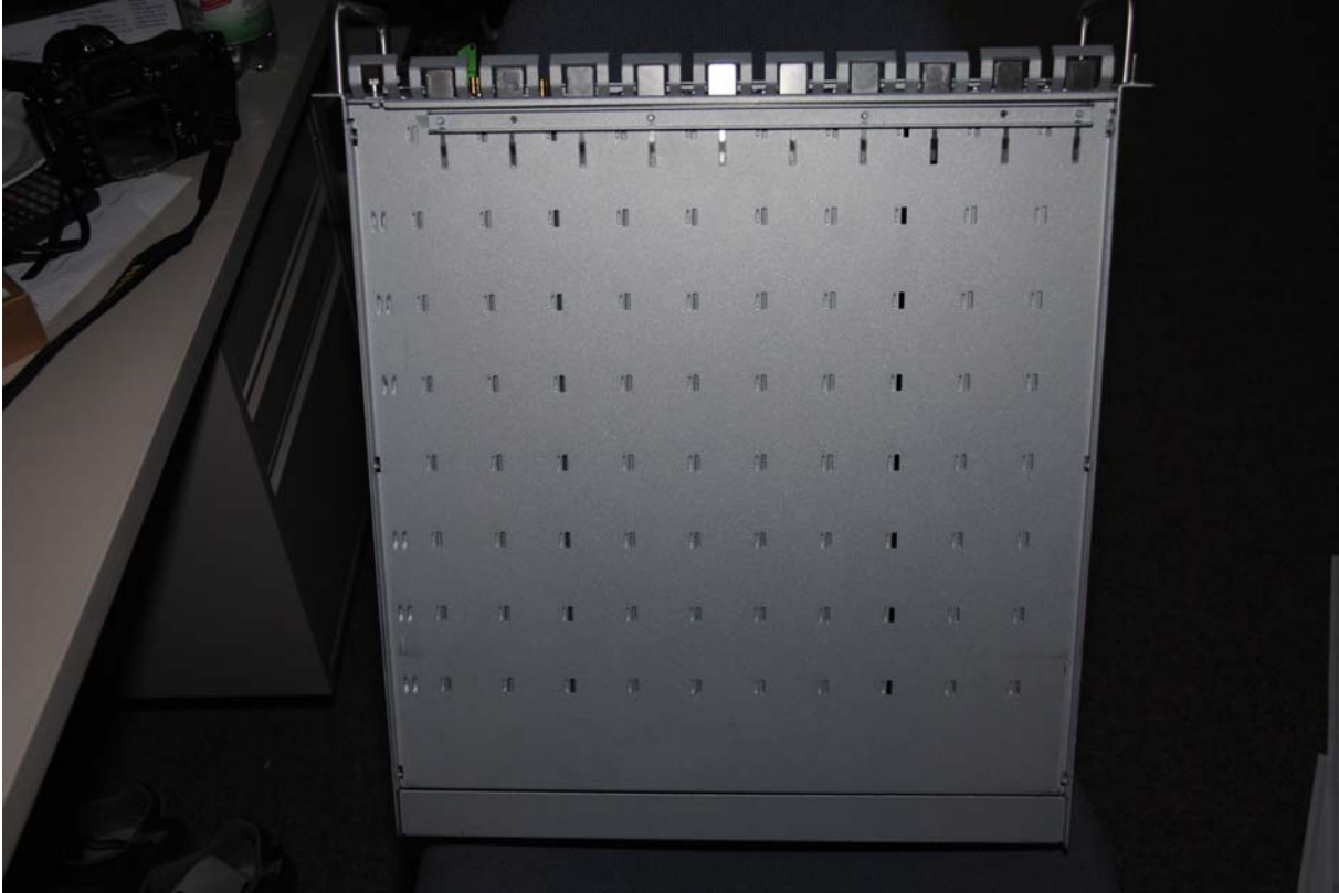
Bottom of first cabinet
