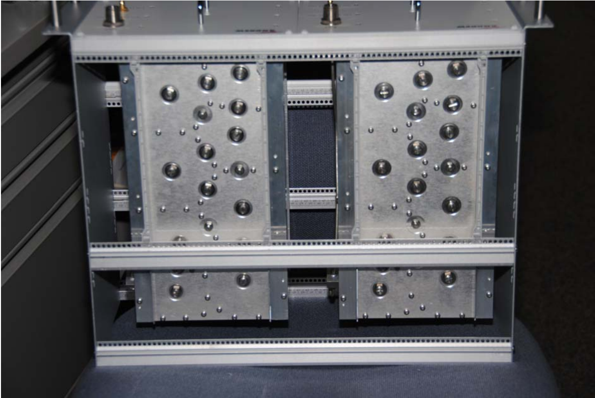
Bottom of third cabinet
