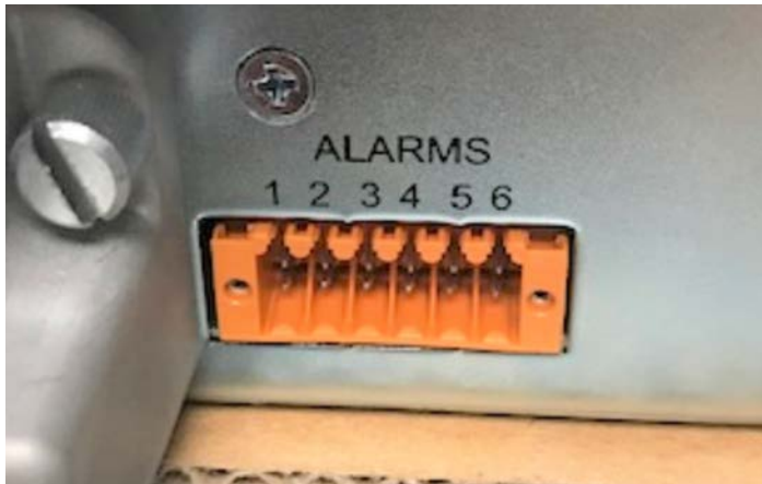
Alarm port on WCS back panel
