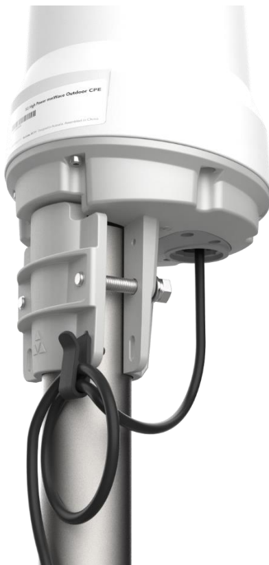
Figure 4 - Ethernet cable strain relief loop
