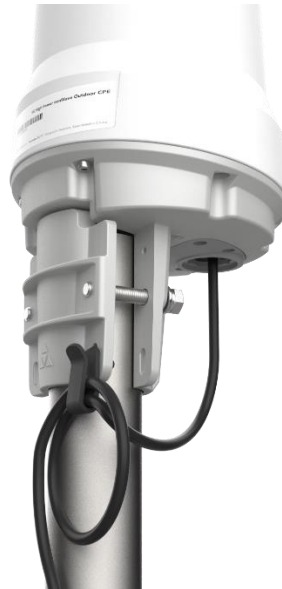
Figure 9 - Ethernet cable strain relief loop
