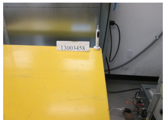
AC LINE FRONT PHOTO
