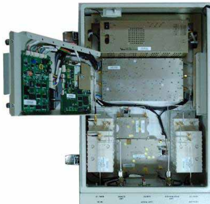
< The Inside of the Repeater >
