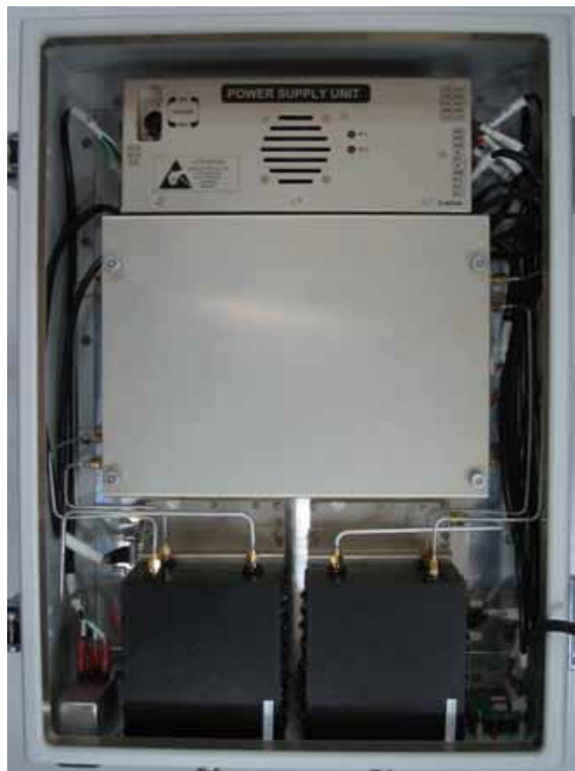
< The Inside of the Repeater >
