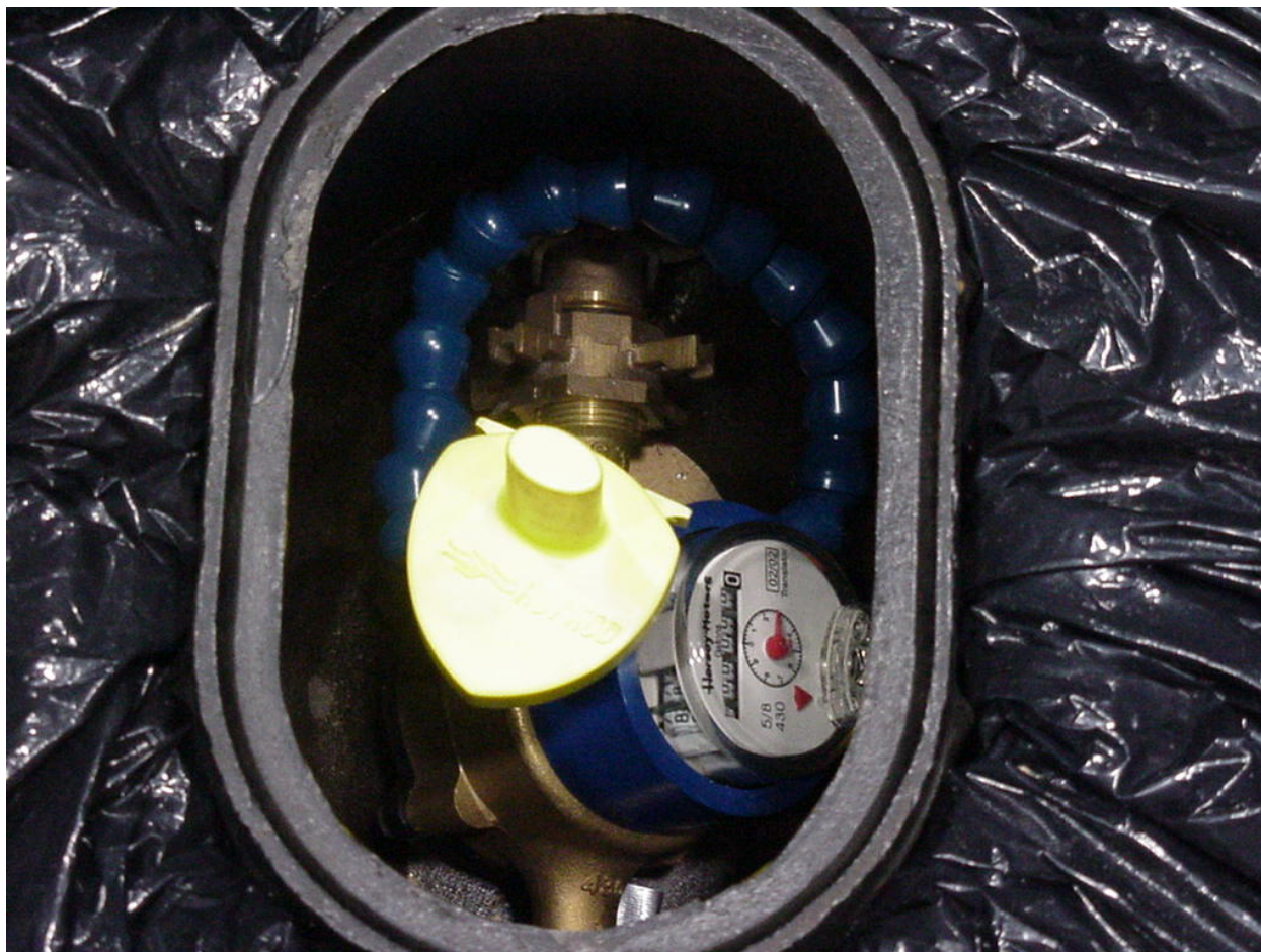
Figure 2 – Photo of EUT Installed in Meter
