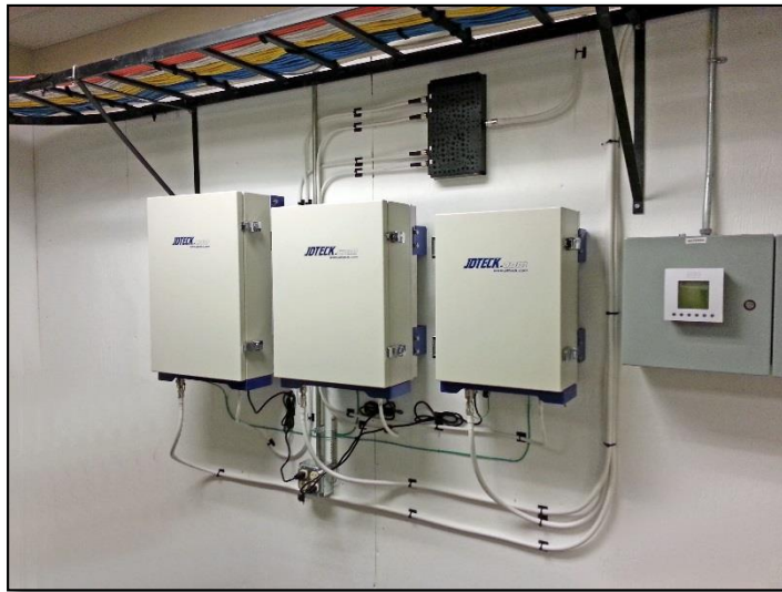
Example of repeaters installed in communications closet.
