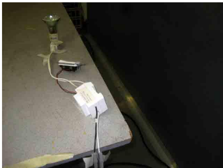
DIMMER, LIGHT OFF
