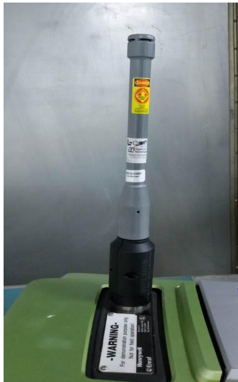
Antenna - 1 with Surge Arrestor
