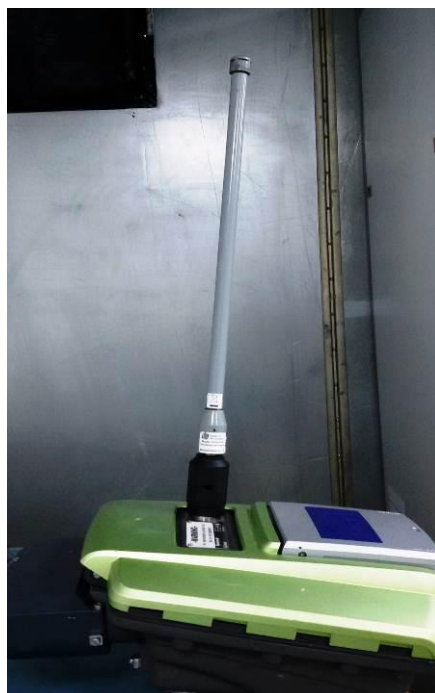
Antenna - 2 with Surge Arrestor
