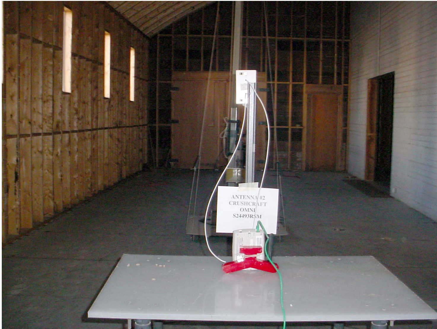
Photo #2b: HiPath Wireless Access Point with Cushcraft Omni, 2 Inputs External Antenna Model: S24493DS, 3 dBi gain
