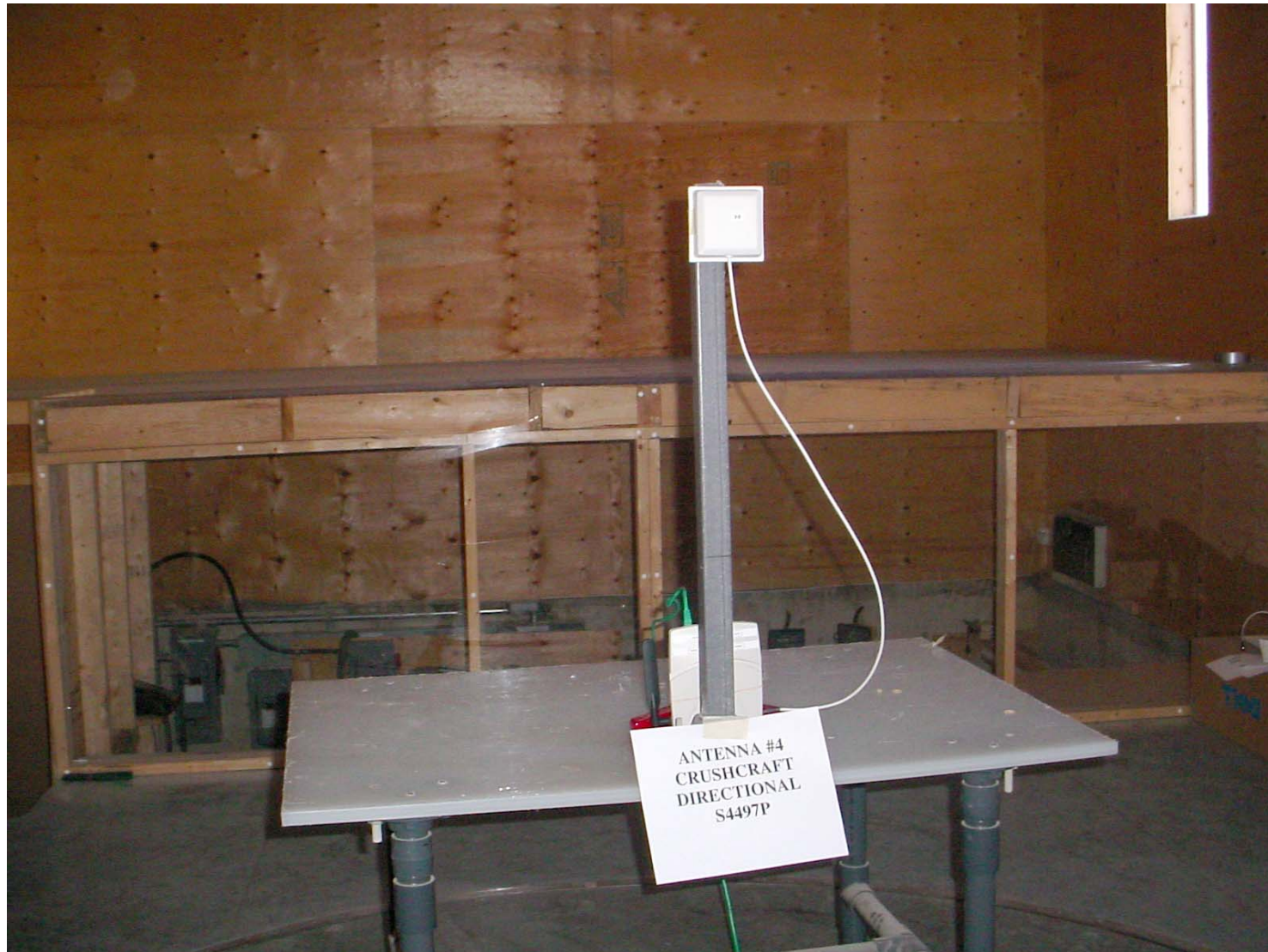
Photo #4a: HiPath Wireless Access Point with Cushcraft Directional External Antenna Model: S24497P, 7 dBi gain
