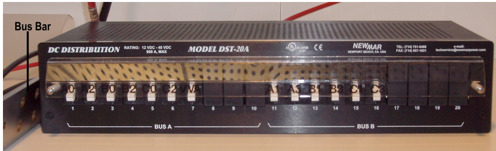
Figure 2.5: DC Breaker and Bus Bar, Front View
