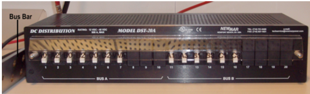
Figure 2.5: DC Breaker and Bus Bar, Front View
