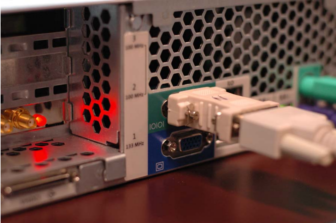
Figure 2: Close-up of a null modem cable connected to the serial console port of the HP ProLiant server.
