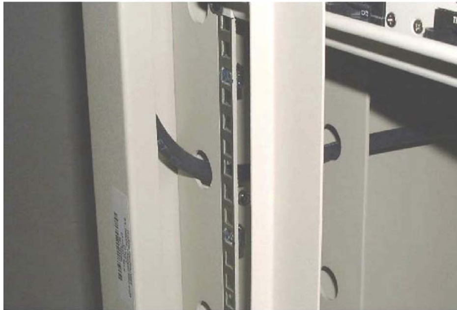
Figure 4.5 Cable Routed Through Structure
