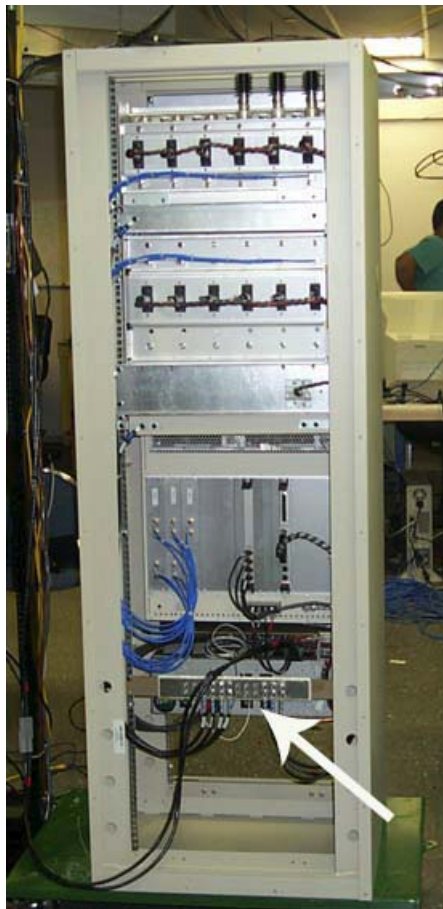
Figure 4.9 Cabinet with Ground Bus Bar — Rear View
