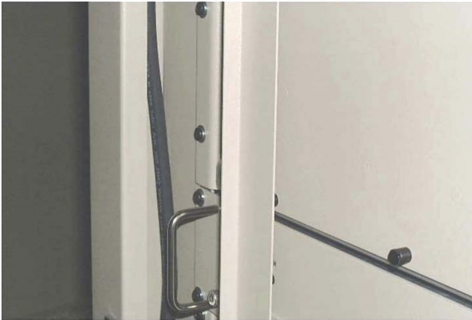
Figure 4.4 Cable Routed in Channel
