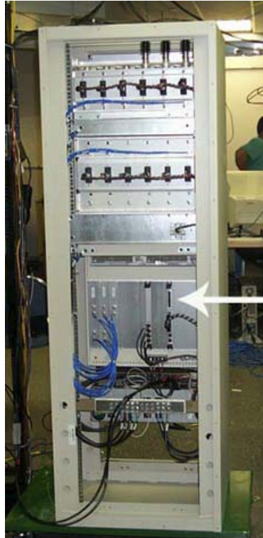
Figure 7.1 Cabinet with Alarm Connection — Rear View
