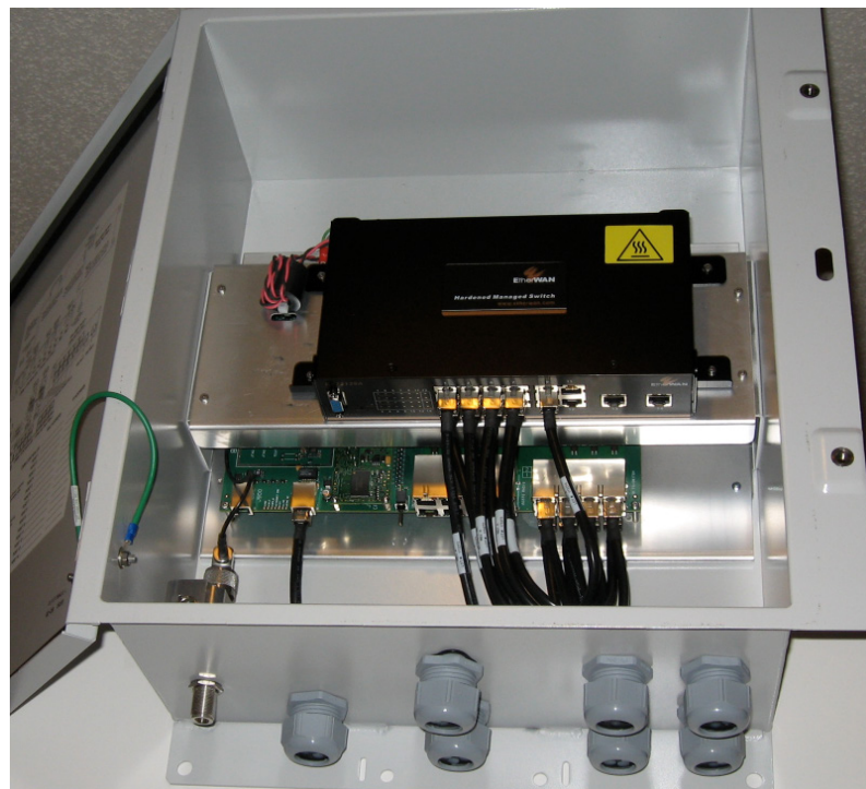
Figure 42 CMM4 (Cabinet with switch)
