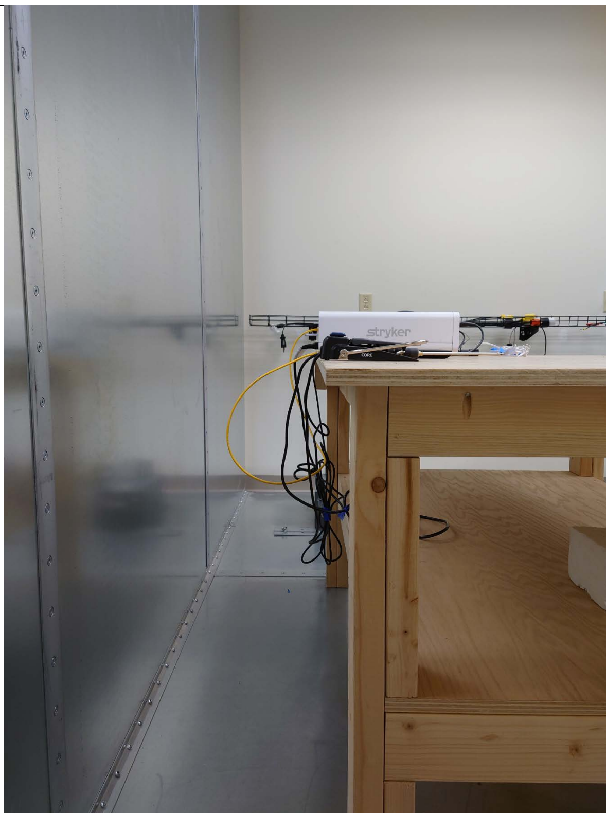
AC LINES SIDE
