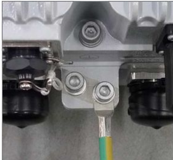
Figure 4-40 R8882 Grounding Bar Connection
