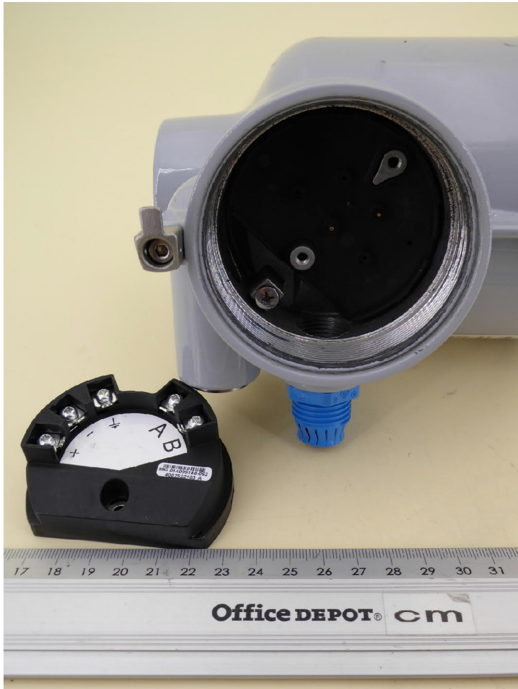
Internal view, terminal board removed
