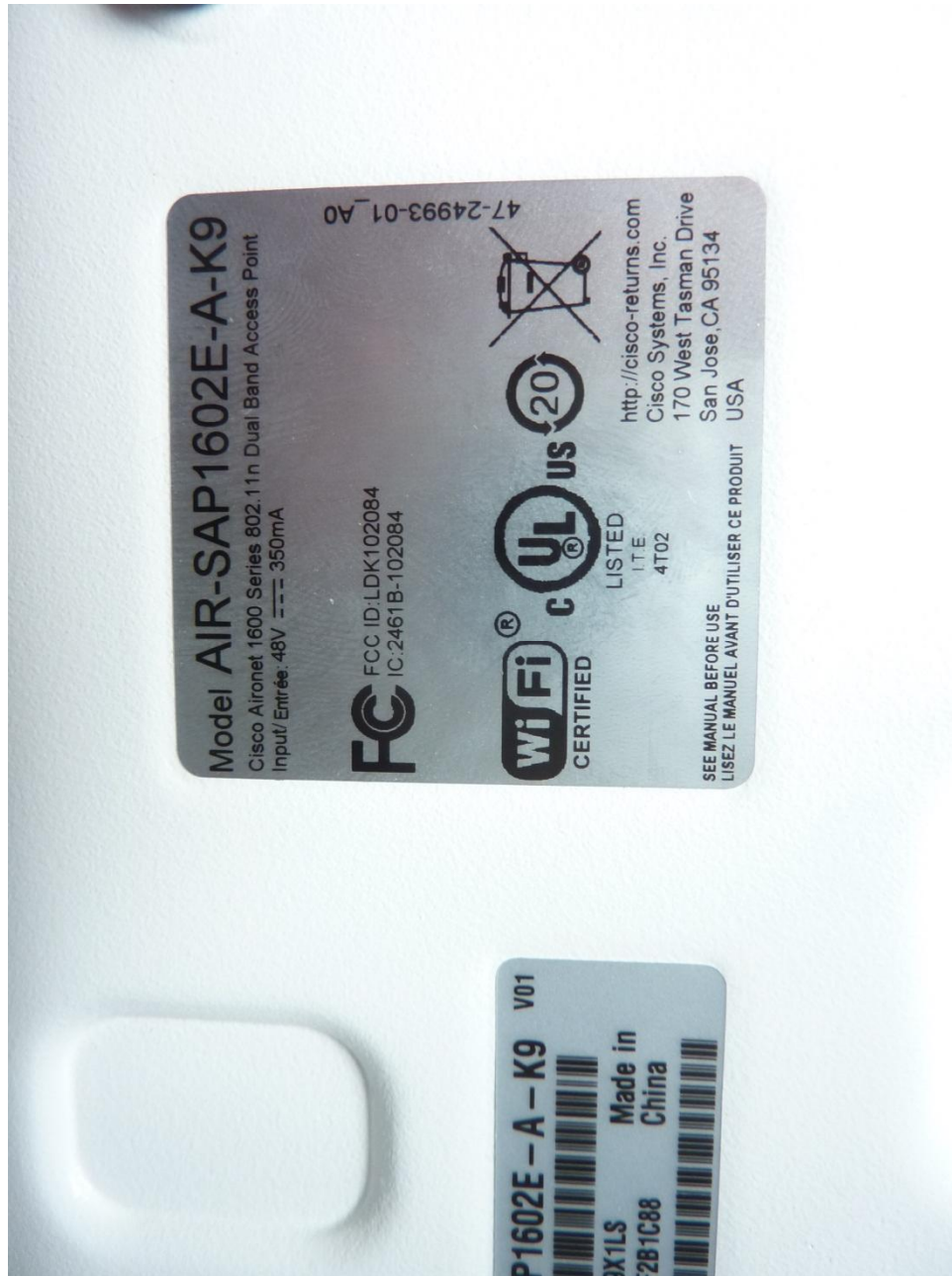
136117_DFS9.JPG: Type plate Cisco Access Point
