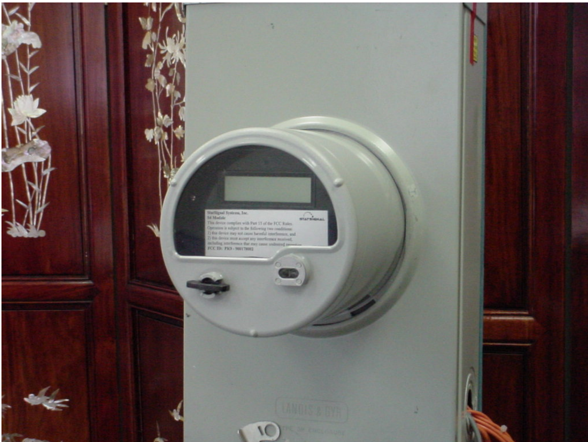
Photo One – External Electric Meter & Housing, Showing location of FCC ID Label
