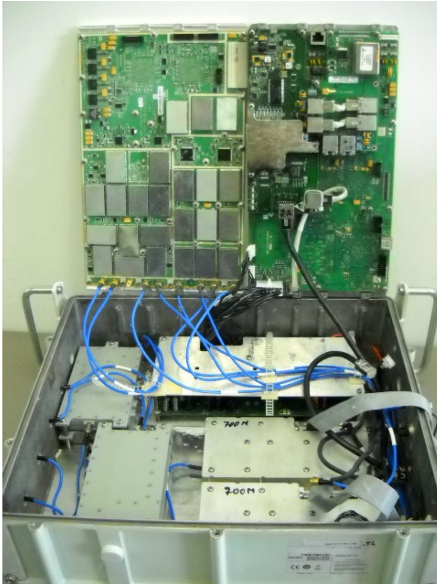
Photograph No.1 “MacroMAXe 0707 700M Ext” internal view
