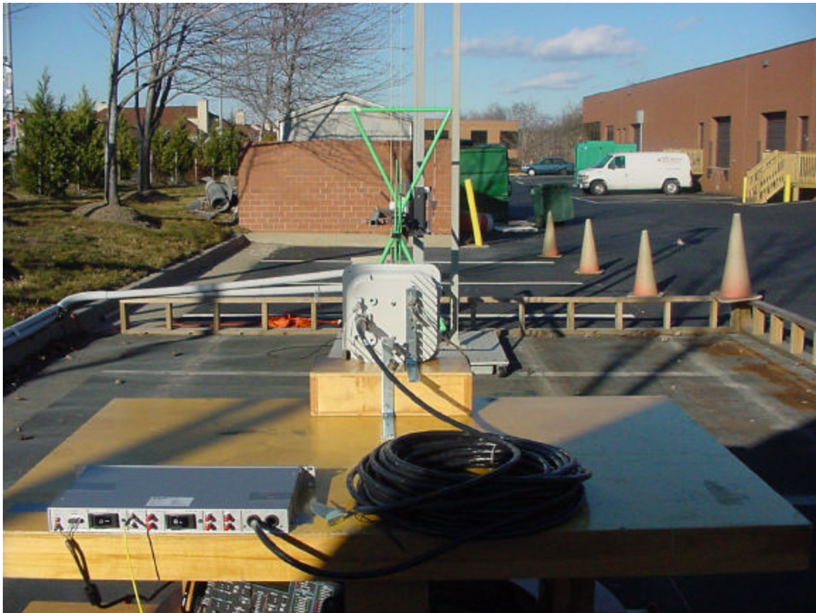
PHOTOGRAPH 2: CONFIGURATION OF TESTED SYSTEM (REAR VIEW)
