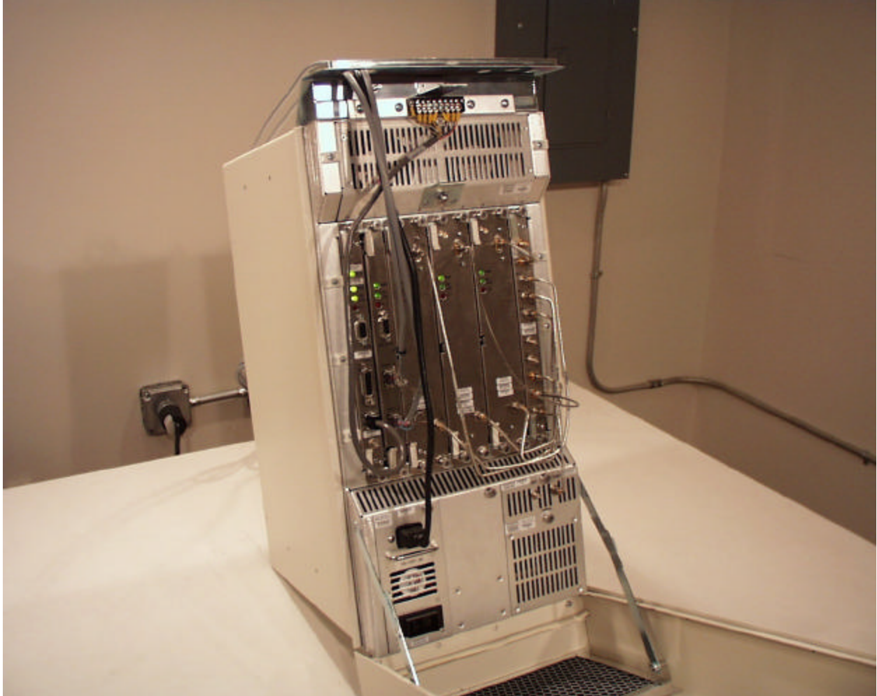
Inside view of the M5324/2
