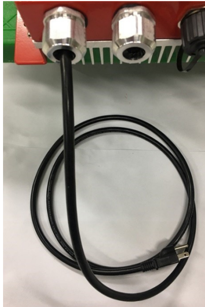
Figure 5-9: Power Cable Connected to Signal Booster
