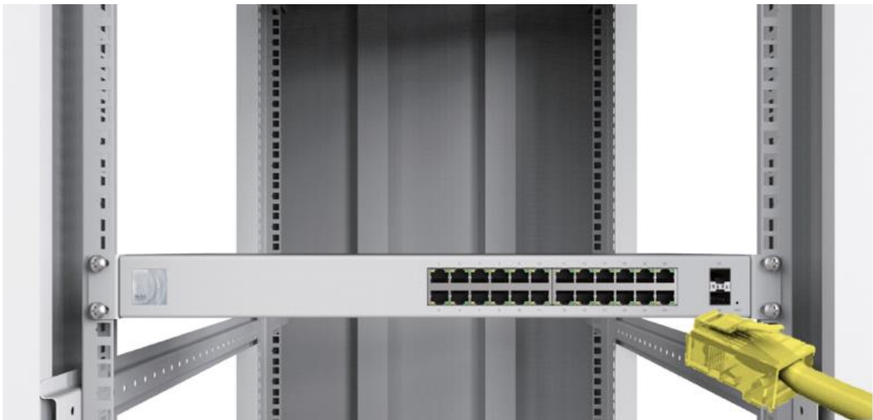
FIGURE: Ethernet cable connection
