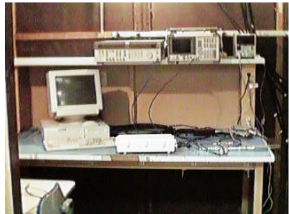
Figure 4 - Sub station setup (PC & SkyWay unit) with test equipment
