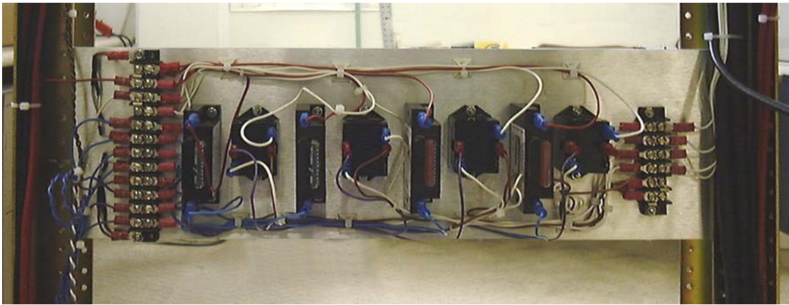
Figure 11. Power-on Delay Panel.
