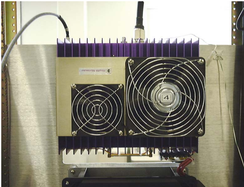
Figure 14. Power Amplifier (1 of 4).
