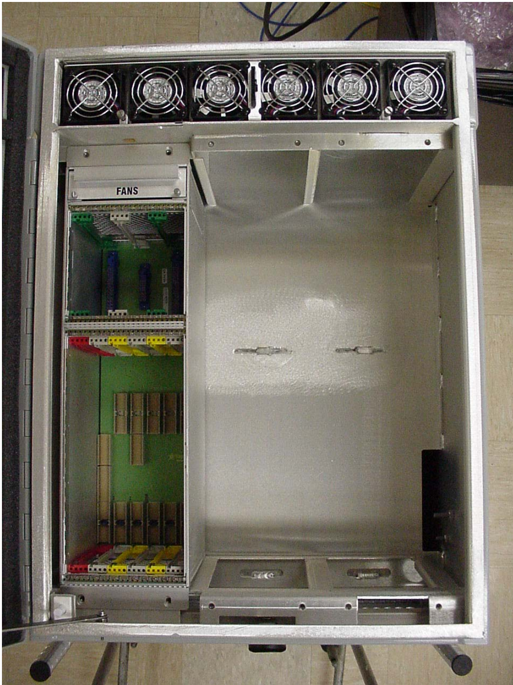
RAN Disassembly - Empty View - Closeup
