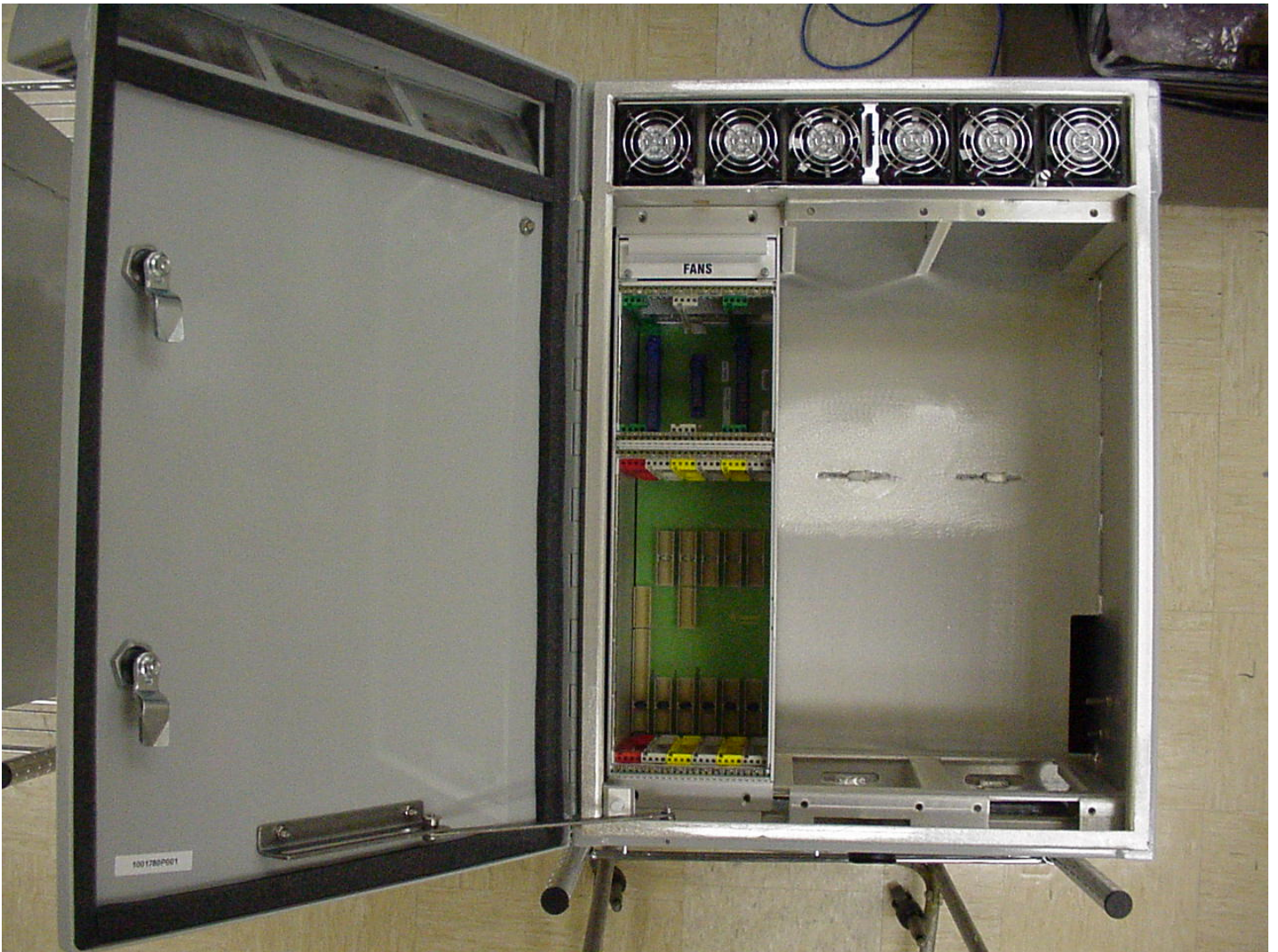
RAN Disassembly - Empty View
