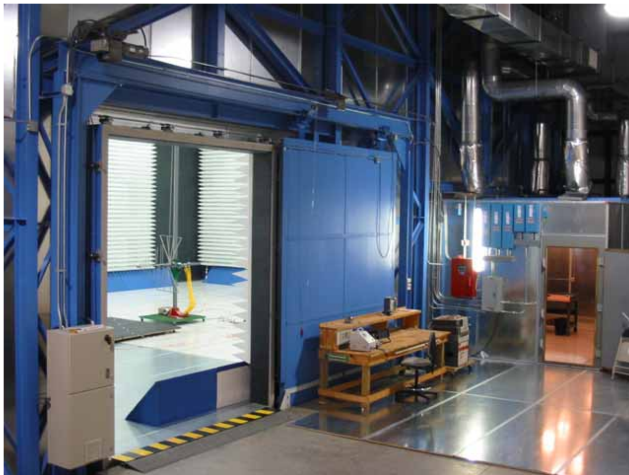
Figure 3-1: 10-Meter EMC Site
