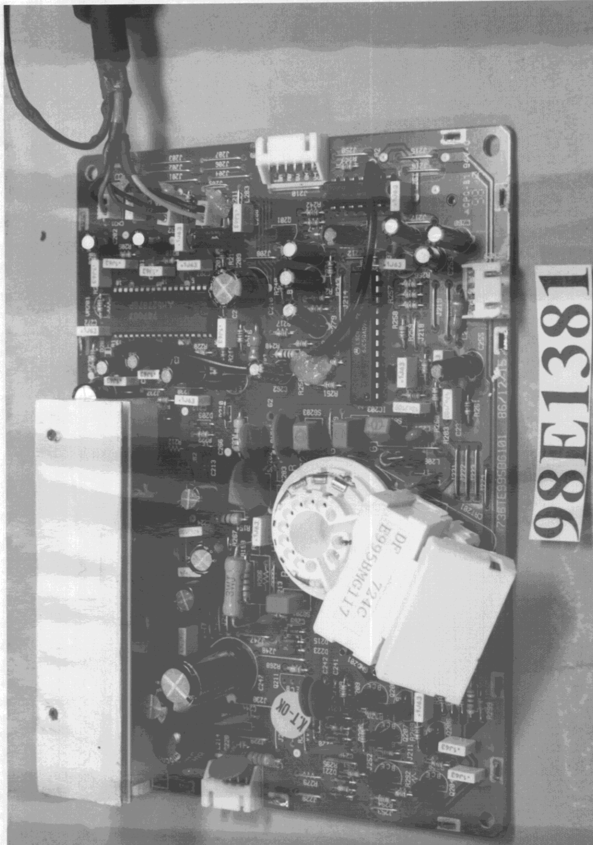
Photo # 16. Unit Partially Disassembled
