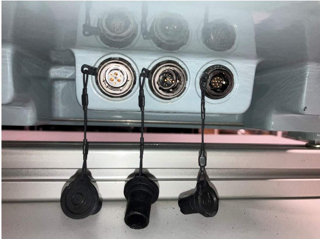
External - Close up of Connectors
