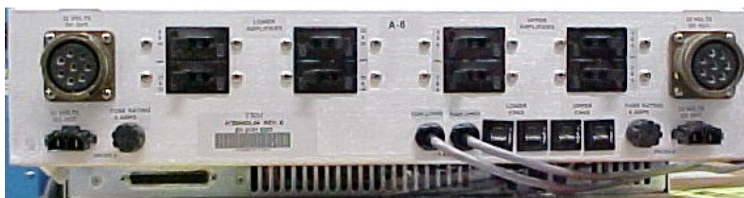
Figure 12 Front-end 48VDC rectifier system (rear view)
