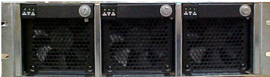
Figure 11 Front-end 48VDC rectifier system (front view)
