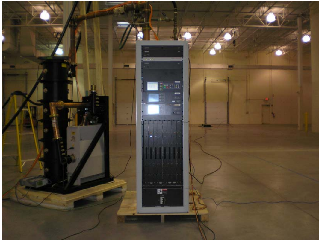
Transmitter and Filter in test room
