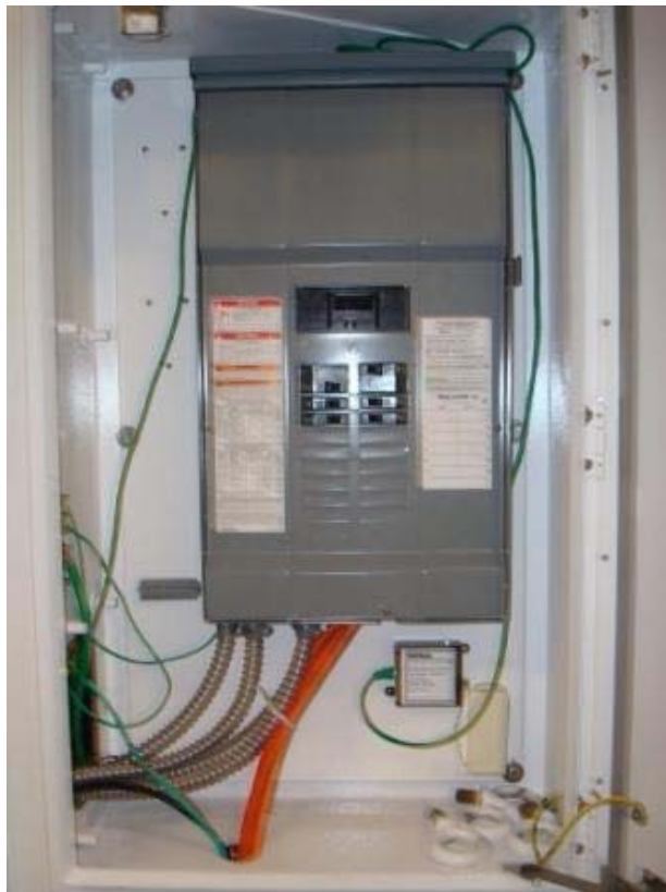
Figure 20, Circuit Breaker Panel
