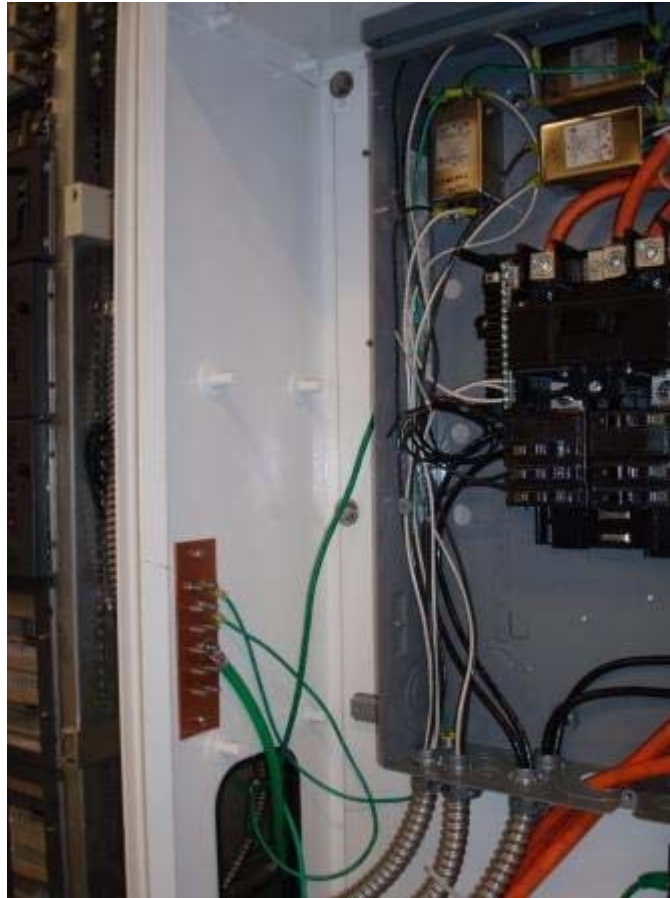
Figure 23, Circuit Breaker Panel Ground
