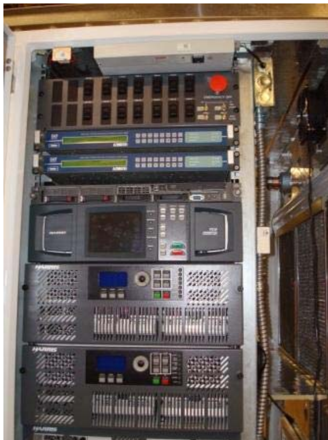
Figure 26, Breakers, Demods, TCU, Exciter
