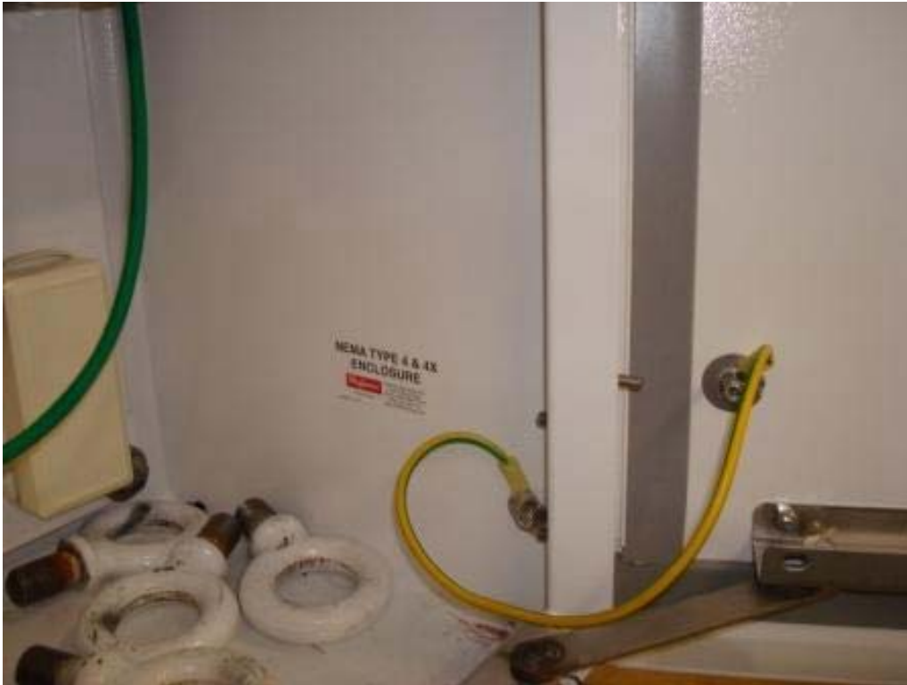
Figure 21, Circuit Breaker Door Ground
