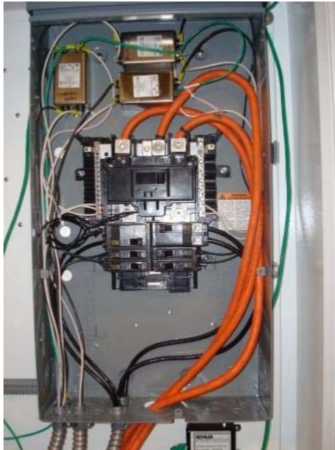
Figure 24, Circuit Breaker Panel Open
