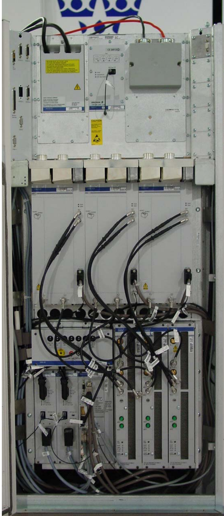
RBS 2207, Open door view
