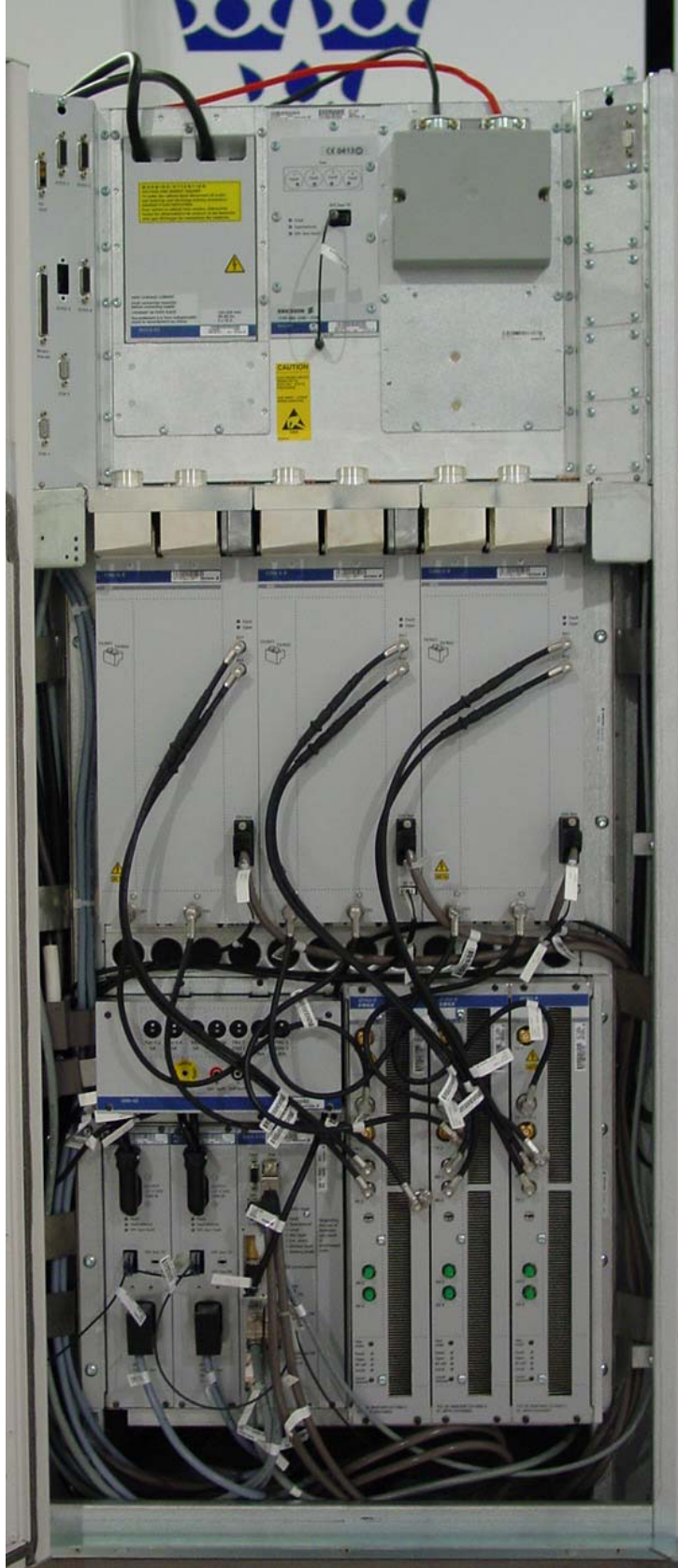
RBS 2207, Open door view
