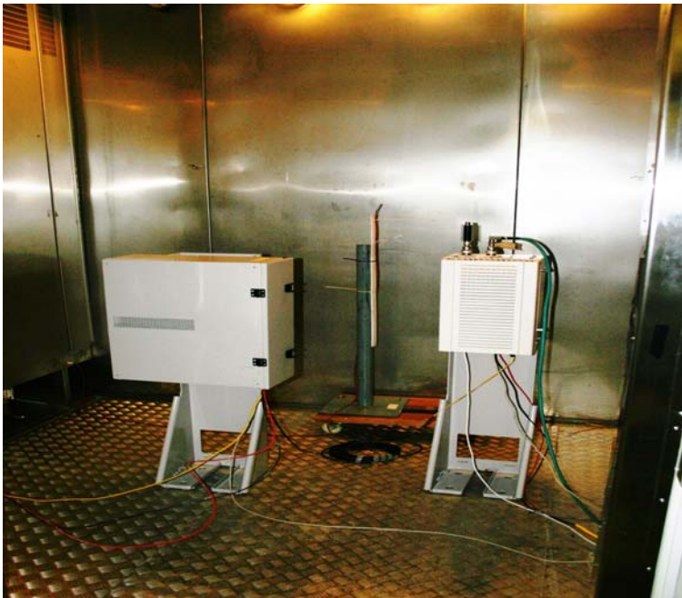
Figure 10.2 1900RRH and BBU mounted on test stands.
