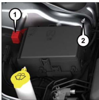
Remote Battery Posts
