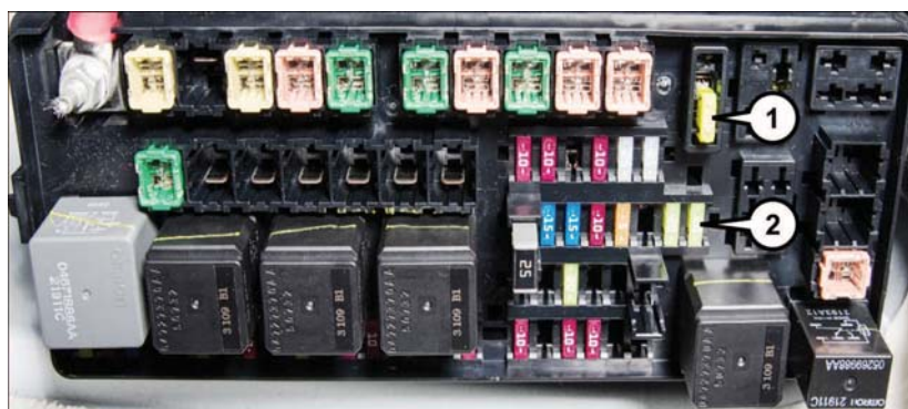
Power Outlet Fuses
