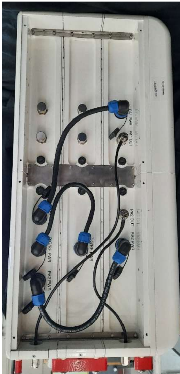
Left Side – Cover Removed
