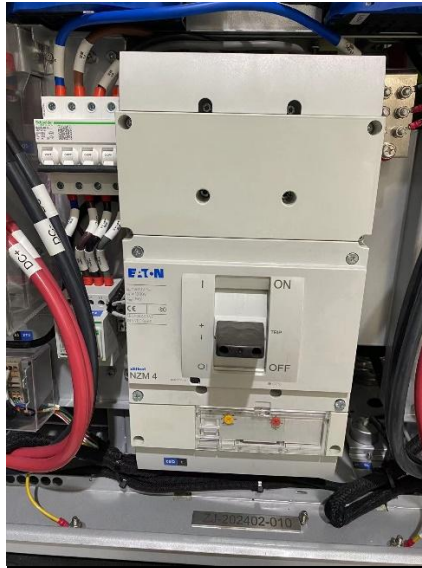
Figure 27 Main switch location
