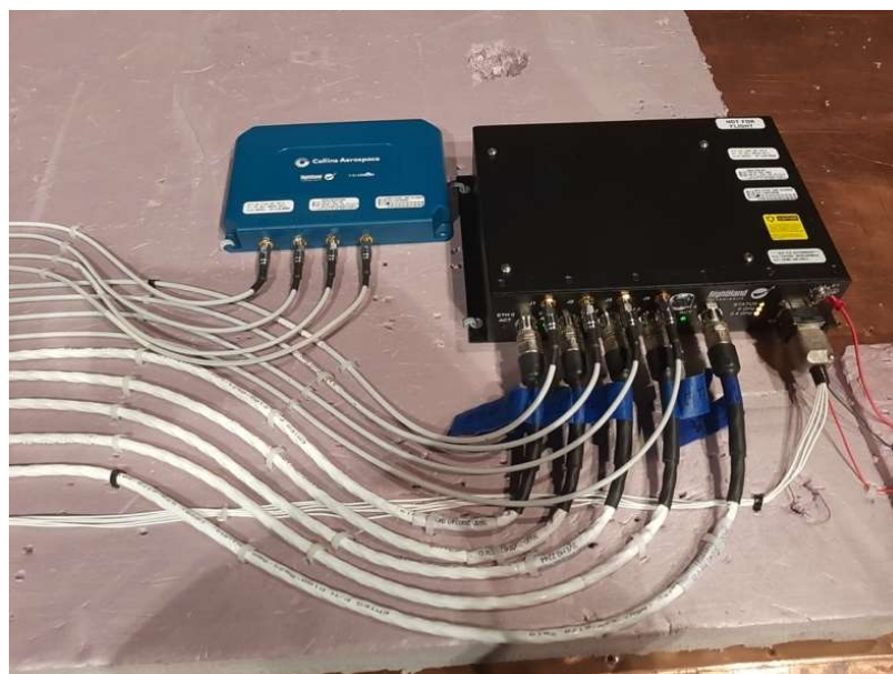
CabnLink Antenna Cabling
