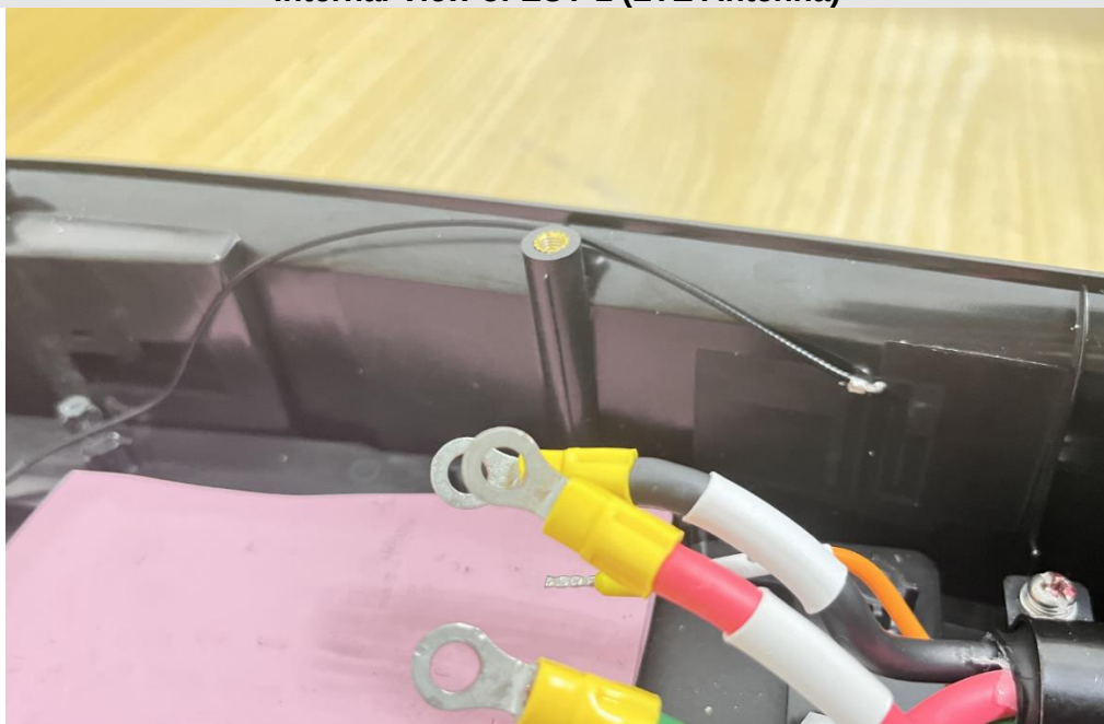
Internal View of EUT-2 (LTE Antenna)
