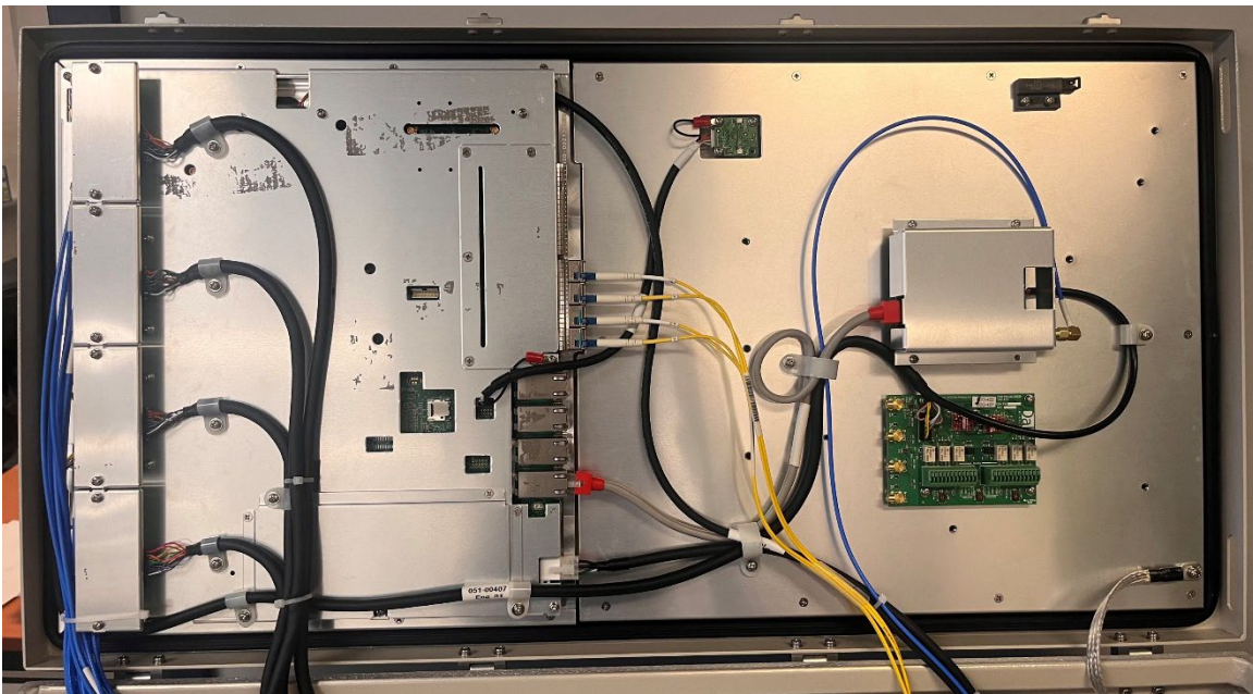
Figure 22: internal view of the cover of RU37-4-PS-ABGH-41-C-D0-2C
