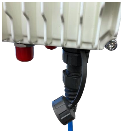
Figure 36: Ethernet Cable Connection to GM02
