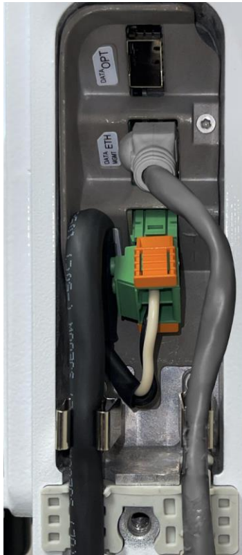
Figure 46: Mesh AP Wiring Cavity Cabled
