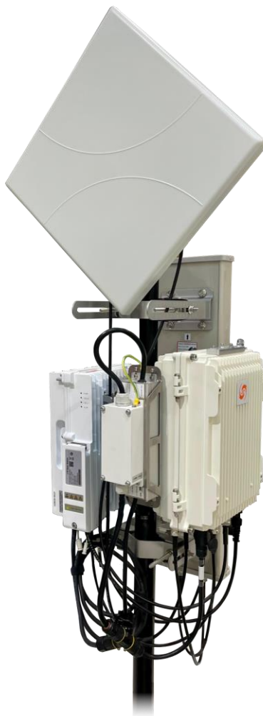
Figure 4: Pole Mounted GM02 Mesh Node & G501 Mesh AP with Antennas
