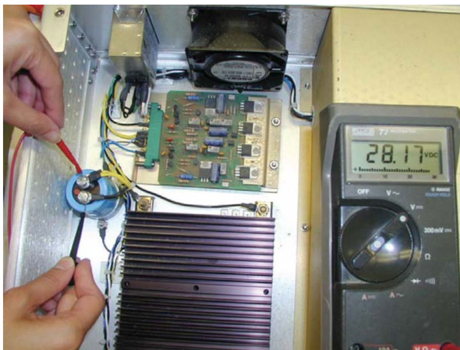
28V DC power supply measurement.
