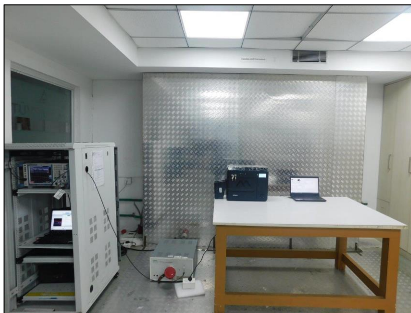
AC Powerlines Test Setup
