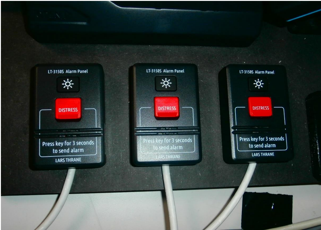
Figure 1.5.4 Alarm Units (Top)
